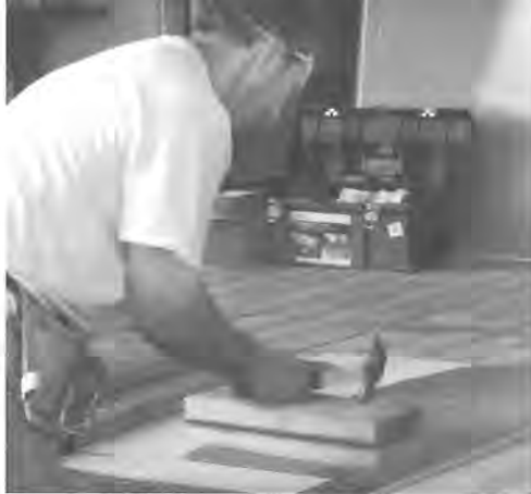
Larry Wittig of Shenandoah District repairs hurricane damage in Citronelle, Ala., as a volunteer with Brethren Disaster Response. The house is just down the road from Cedar Creek Church of the Brethren.
