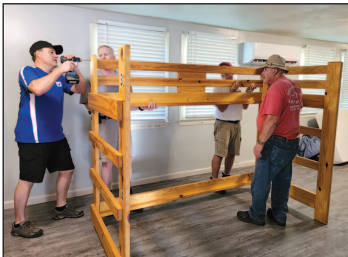
The moving crew worked hard to get the Letcher County, Ky. volunteer housing site up and running. Photo courtesy of BDM
