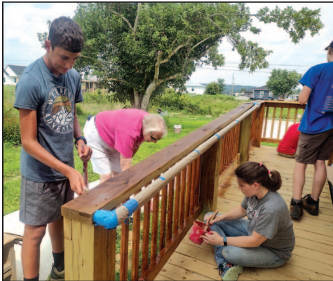
BDM volunteers work to complete Habitat houses for survivors who will become new homeowners in Dawson Springs, Ky. Photo courtesy of BDM
