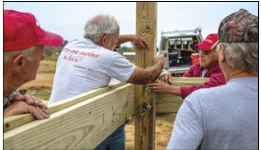
Construction disaster project leader Rex Miller (c) demonstrates the next step in building this deck for a home in Dawson Springs, Ky. by Benjamin Hoffmann
