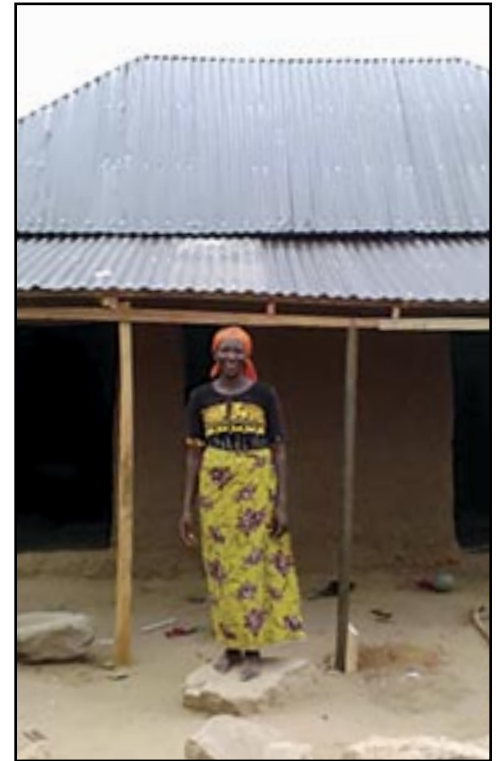
Providing new roofs for repaired houses is a major program of the Nigeria Crisis Response.
