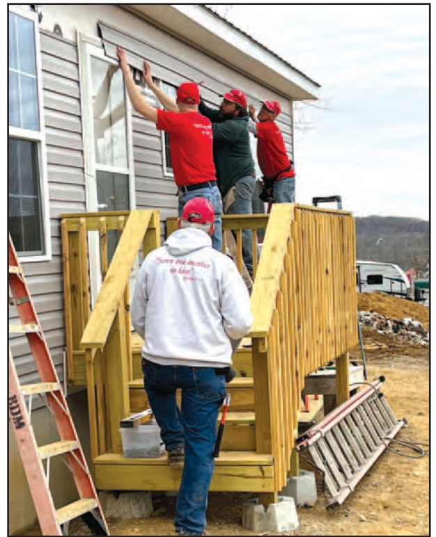
Volunteers install siding on a new home in Dawson Springs, Ky. Courtesy of Troy Barnhart
