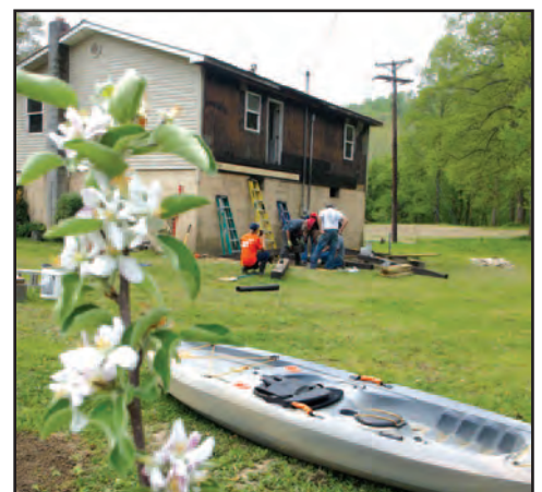
BDM volunteers begin to build a new deck to replace the one washed away in the 2022 storm. The homeowner used a kayak like the one in the foreground to escape the rising flood waters. Photo courtesy of BDM
