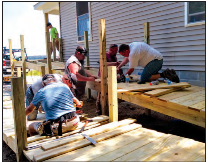
Volunteers built a ramp for a house that was raised above flood level following tidal flooding in Maryland. Other volunteers worked on the inside of the house.
