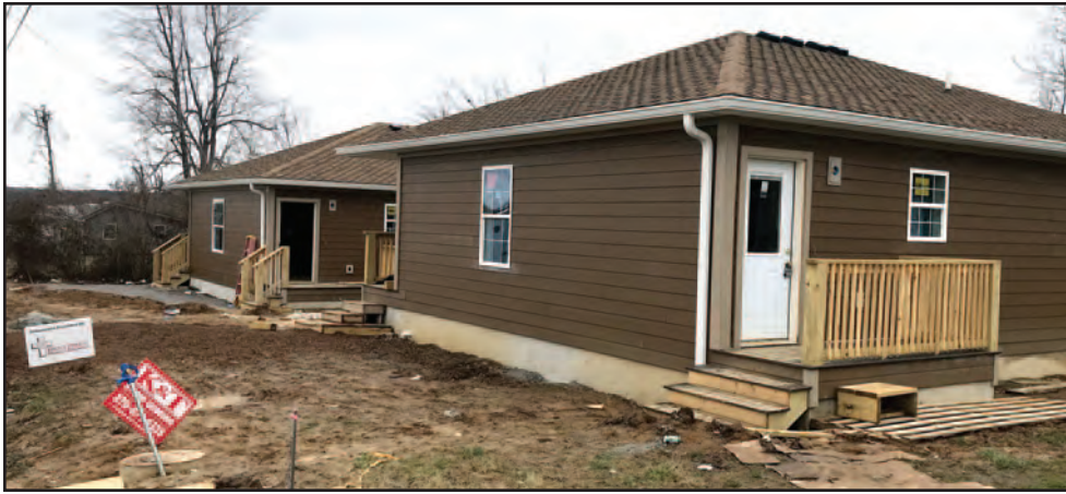
BDM volunteers in Dawson Springs, Ky., are working with Habitat to build new homes to replace houses destroyed during the December 2021 tornados.
