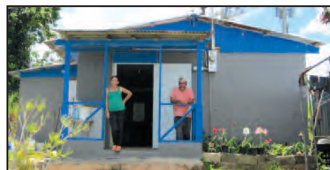
The same Río Prieto house after partial repairs. Photo by Sharon Franzén
