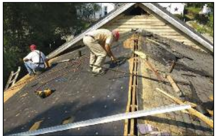
BDM volunteers from South/Central Indiana and Illinois/Wisconsin districts repaired a roof in Ottawa, Ill., damaged in February 2017 by an F-3 tornado. The team worked with the Ottawa/Naplate Long Term Recovery Group, which had formed with support from the Disaster Recovery Support Initiative (DRSI). Photo courtesy of Cliff Kindy
