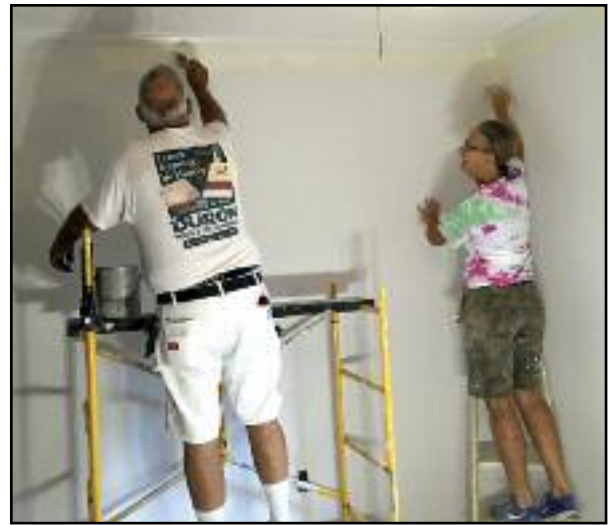
Volunteers paint walls in one of the first homes BDM worked on in Marion County, S.C. Photo by Jenn Dorsch-Messler
