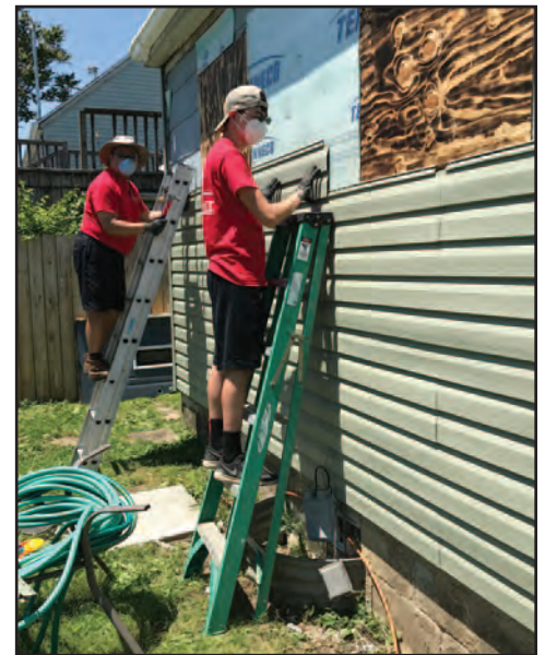
In June 2020, a small group of volunteers from the Southern Ohio/Kentucky district continued outdoor work on a home damaged in a Memorial Day 2019 tornado. Photo by Burt Wolf
