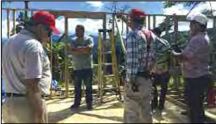
District executive José Calleja (center) visited BDM volunteers working on a new build in Puerto Rico and tearfully thanked them for supporting the church and island in Hurricane Maria recovery.
