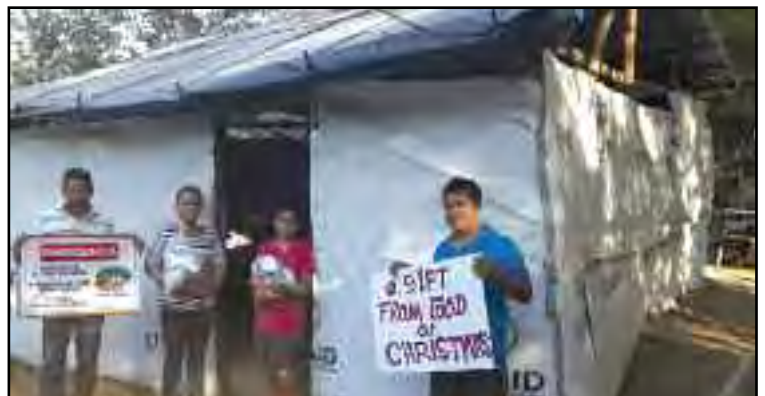
Top: Homeowners repaired their flood damaged homes as best they could. Bottom: An EDF grant brought assistance—just in time for Christmas.
