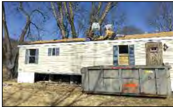
Volunteers repair a roof in a trailer park in Eureka, Mo. Families whose own trailers have been continually damaged in repeated flooding are being moved from the floodplain to repaired homes in this new location. Photo by Jenn Dorsch-Messler
