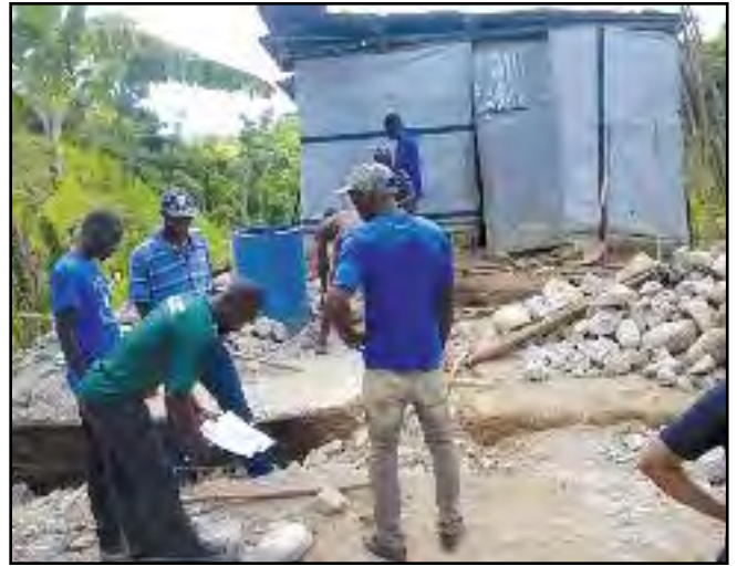
Hurricane Matthew recovery continues in Haiti with home reconstruction. Working in partnership with the Haitian COB, BDM is supporting the repair or rebuilding of 40 homes damaged by the 2016 hurricane. In this photo preparations are underway to build a house for a family currently living in makeshift housing.
